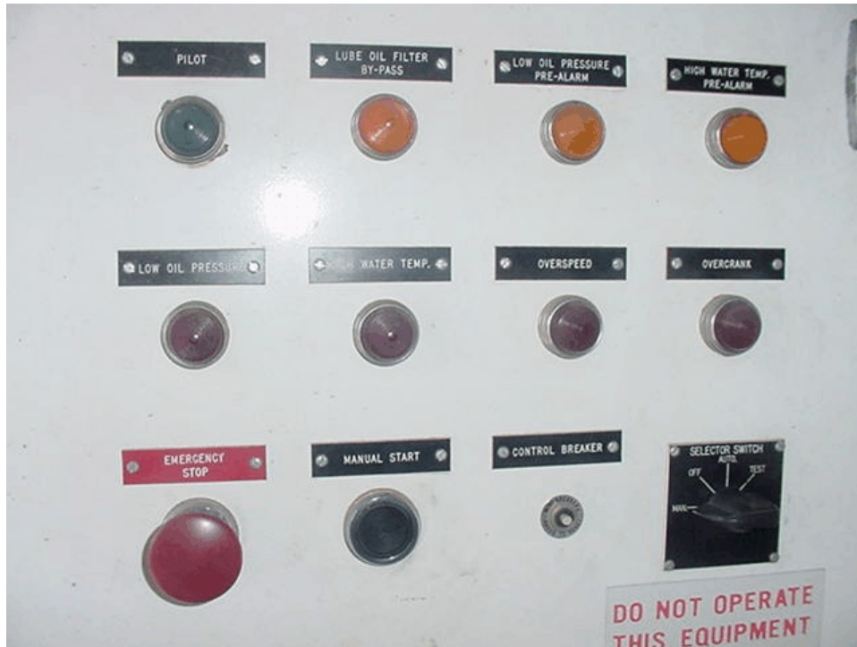
Figure 6. Control Panel – Left Side
