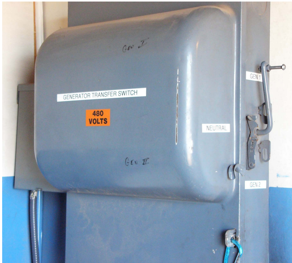
Figure 4. – Generator Transfer Switch
