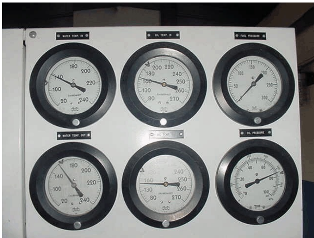
Figure 10. Operating Gauges – Right Side
