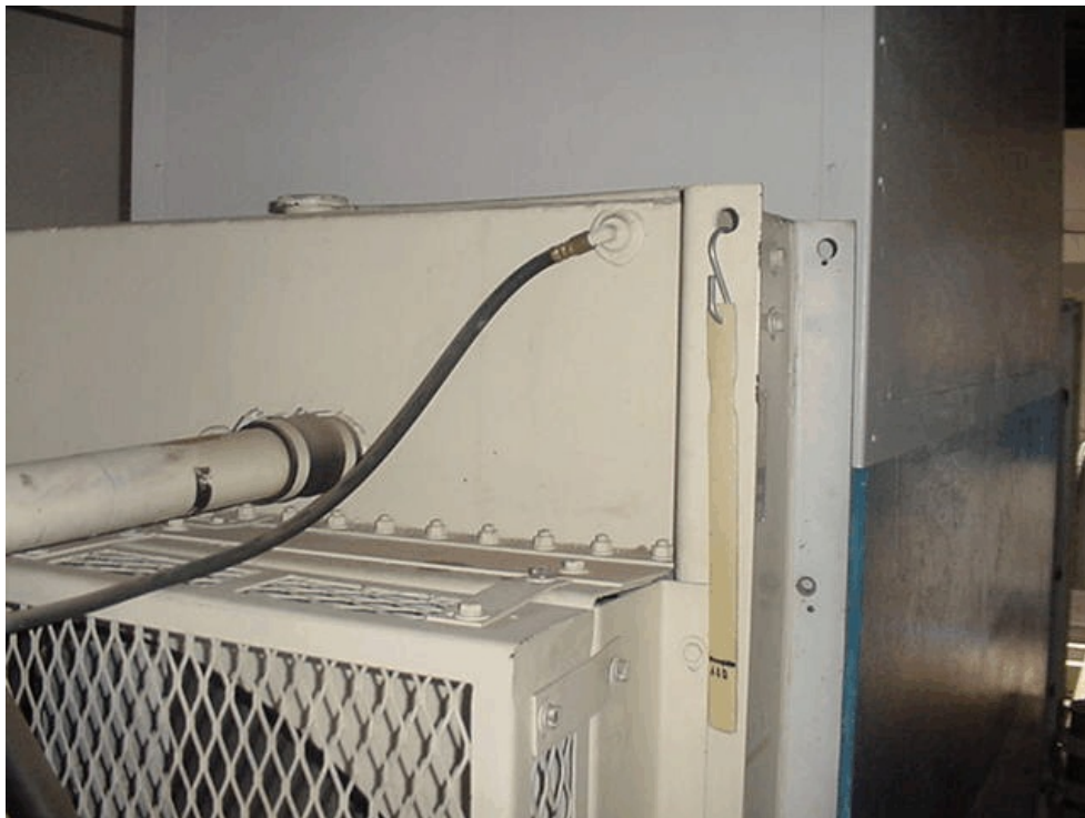
Figure 2. - Water Level Check
