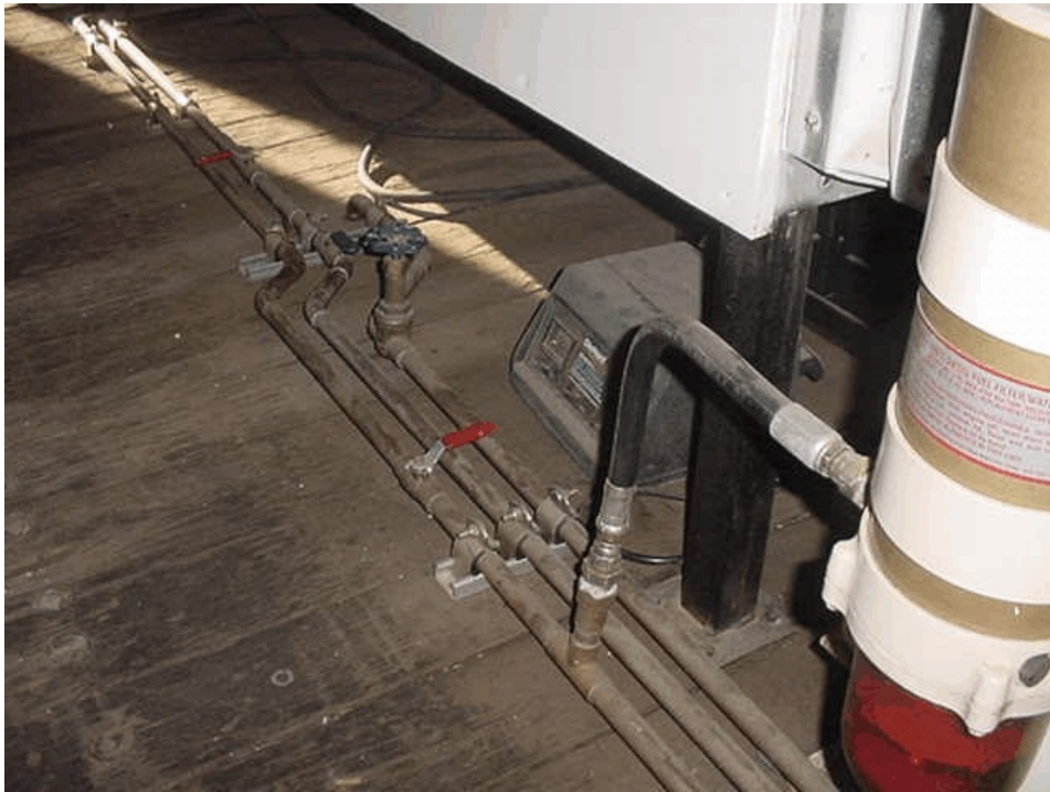
Figure 5. Fuel Shutoff Lines and Valves
